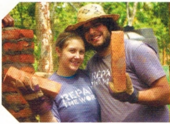
Megan Halliday, left, takes a break from laying bricks for a new educational facility for farmers in Nicaragua.
