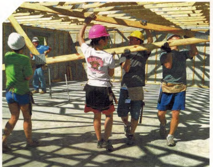
George Jin, far right, works with other Clark School students to construct a roof on a new Habitat for Humanity house in Fort Lauderdale.
